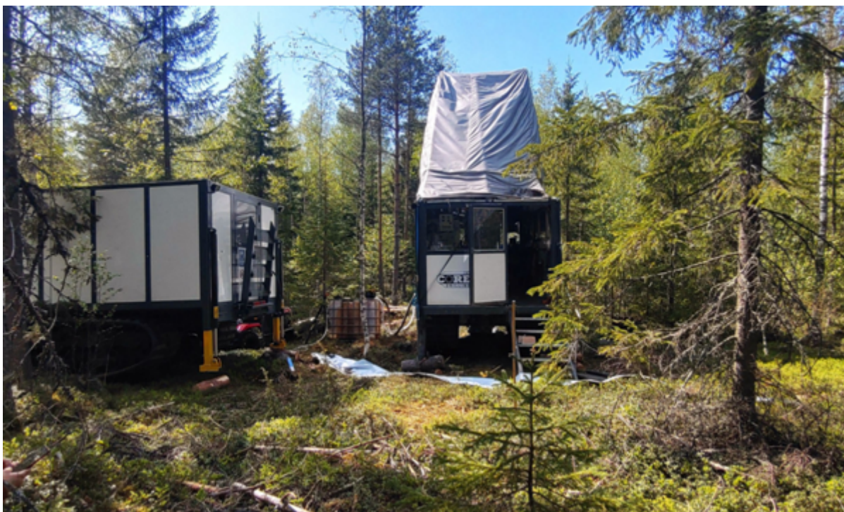
Figure 2: Drilling has commenced at the Hammasslahti Project. Experienced Finnish drilling contractor, MK Core Drilling Oy, were selected to undertake the Programme.
