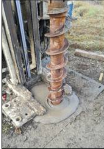
Figure 2: Damaged direct push bit (left), sand liquefaction and escape (right)
