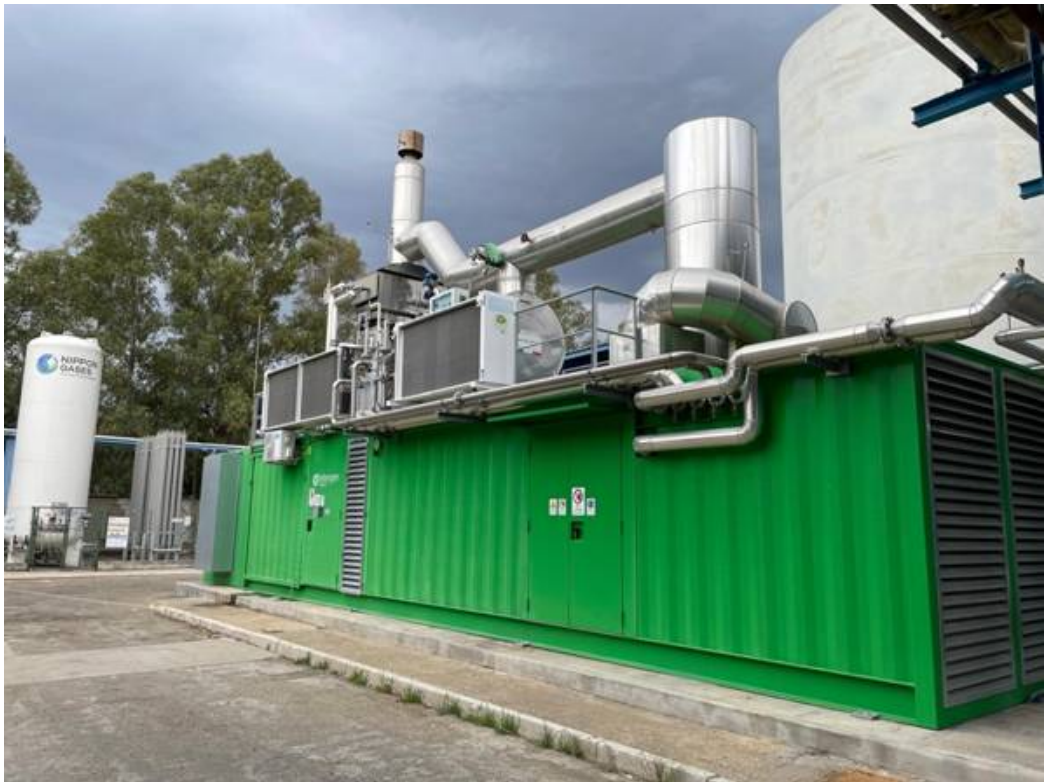
Figure 4 Onsite cogeneration and backup power capacity.
