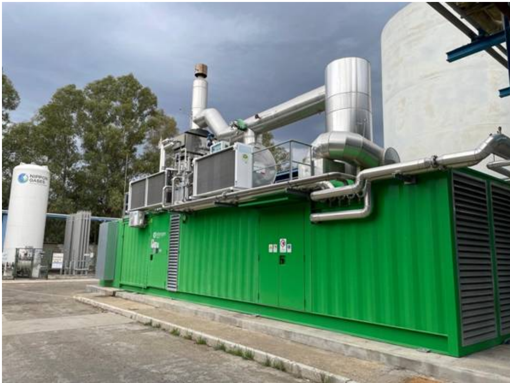
Figure 4 Onsite cogeneration and backup power capacity.
